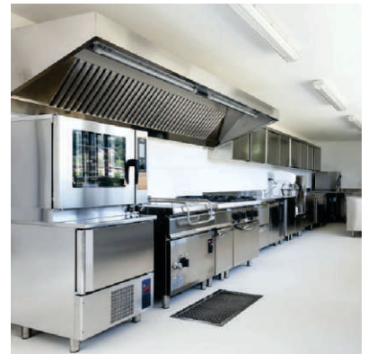
KITCHEN VENTILATION SYSTEM
