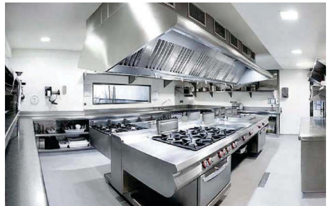
COMMERCIAL KITCHEN SETUP
