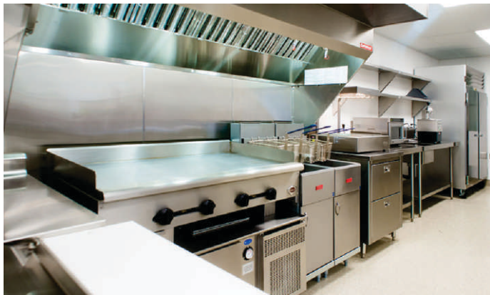
COMMERCIAL KITCHEN SETUP
